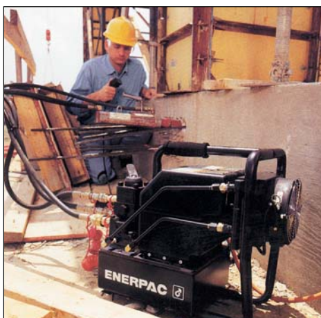
◀ This Titan HD pump is used to power a double-acting post-tensioning cylinder on a construction site.
