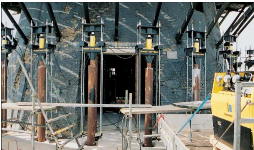
▼ Part of the Dutch Deltaworks: Step-by-step stage-lifting a windmill over a total height of 6.5 feet using 28 Enerpac RR-506 double-acting cylinders powered by three electric pumps.
