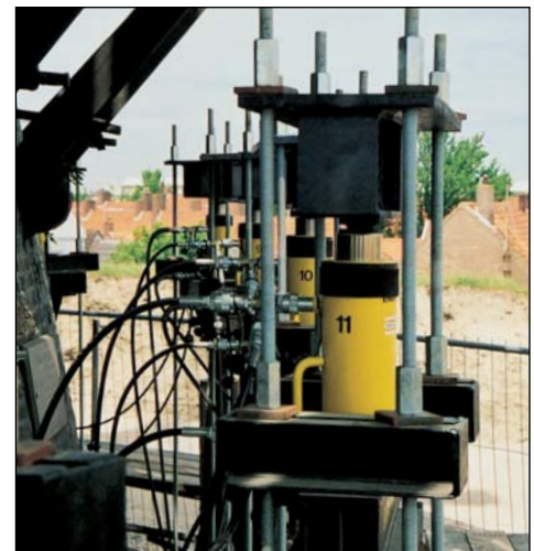
▼ Each cylinder is attached to threaded rods and a supporting column to lift the load of the windmill.
